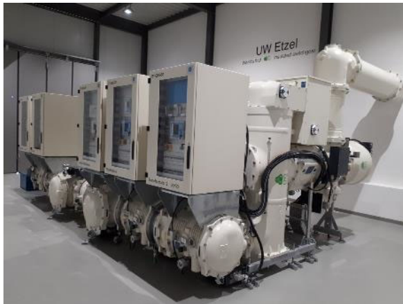
Source: Think Grid article on world first C4-FN substation testing at 145 kV, 2017
